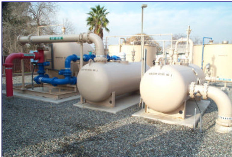
Photo 1 – Typical Filtronics filter vessel (behind blue & red piping) and reaction vessels. Note sodium hypochlorite chemical oxidant injection point (foreground right) and backwash reclamation tank (right background).
