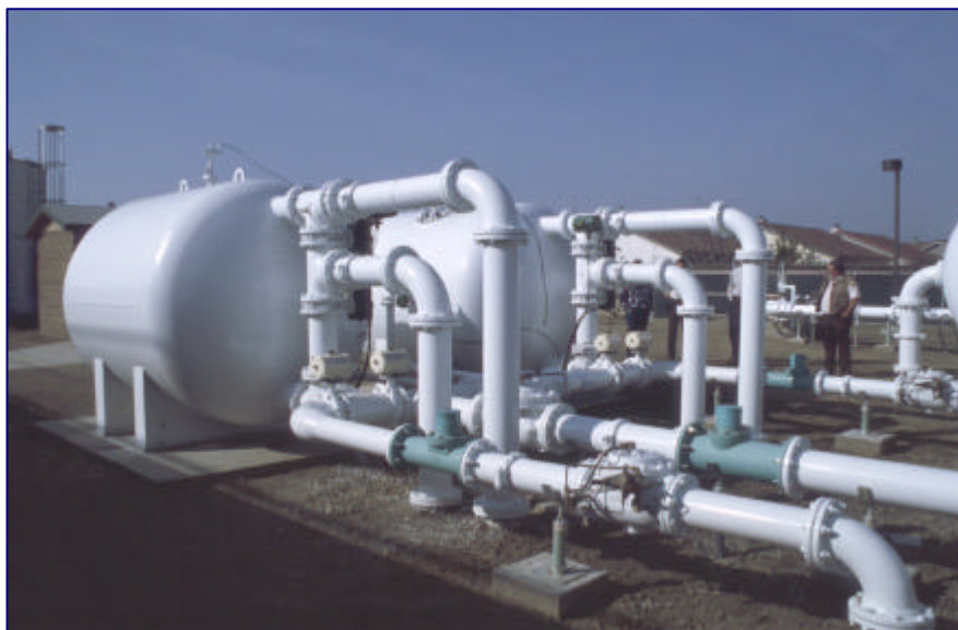
Photo 2 – City of Hanford, CA Filtronics arsenic treatment system
