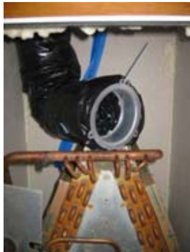
Figure 2-3 Fresh air intake duct sitting atop the cooling coil
