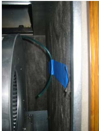
Figure 2-5 Pressure probe at air handler fan
