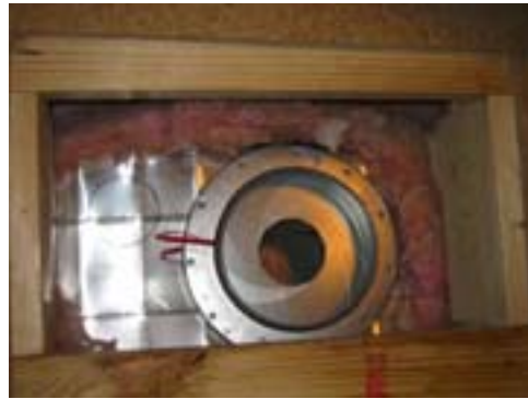
Figure 2-11 Damper in trunk duct of the single section home
