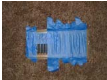
Figure 3-13 Masked air supply register in small bathroom, single section home
