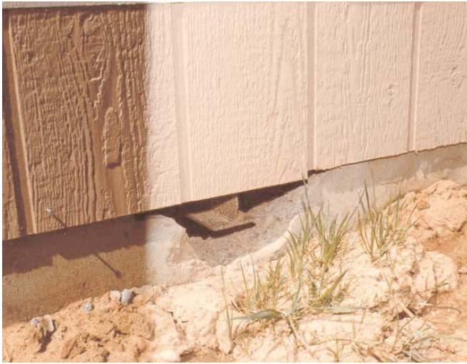
The unattractive exposed I-beam is the result of not recessing the chassis and not providing an adequate trim detail.
