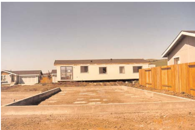
This fully-formed concrete perimeter wall with interior chassis supports is fully recessed (dug out). Backfilling will happen after the house is rolled on.
