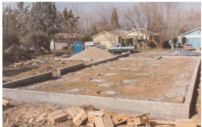
This foundation has a perimeter wall and interior pier supports. It is not recessed because of the lot's excessive upslope relationship to the street.
