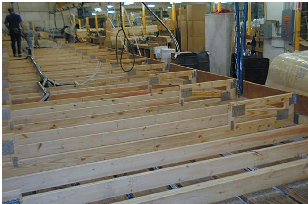
The underside of a floor prior to installation of the bottom board and frame at Wick Building Systems.
