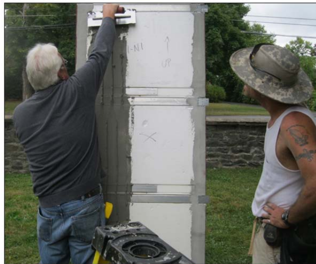
Applying the adhesive to the back of a panel using a notched trowel. Vertical notches allow any water that gets behind the panels to drain down to exit at the bottom of the wall.
