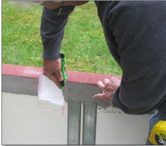
Removing some foam from the back of the panel to accommodate the sill.
